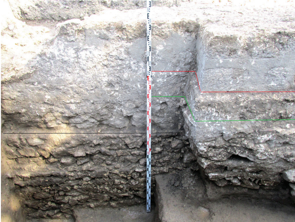
Fig. 16. Mortar coating of the joints between the stone blocks of the face construction of the so-called upper part of the substructure of the widening along the section of the north fortress wall surveyed in 2018–2019 (after ТРАЙКОВА 2024, 140, фиг. 11)
